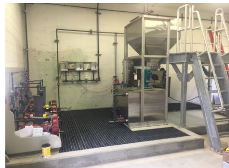
Hydrated Lime Feed System
